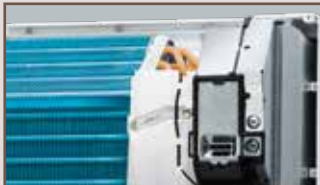
Ensure its reliable operation and preventing fire accident in case of short circuit.
